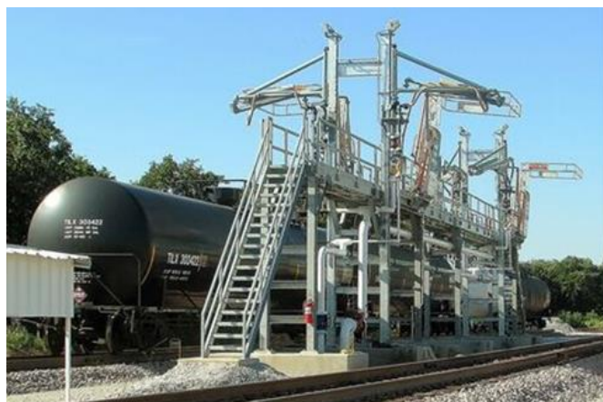
Railcar Rack NGL Thackerville Liquids Terminal
